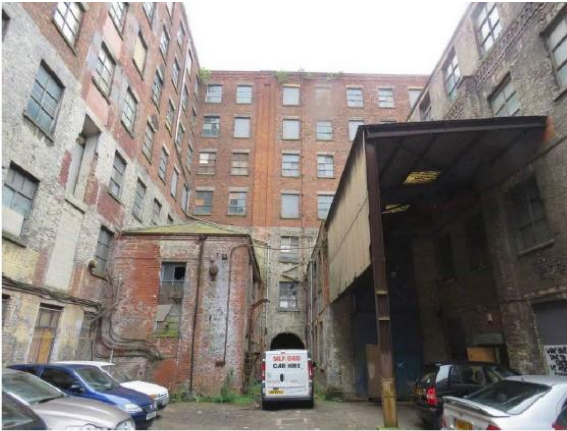
View from within the courtyard including transformer building (left)
